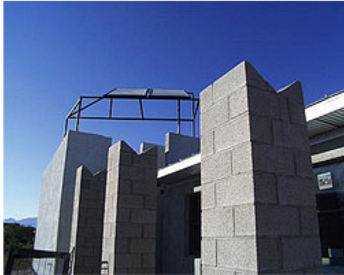
The solar water heating flat plate collectors/shade structure prior to the installation of the rainwater harvesting aqueduct. Photo by Wilson Graham.
