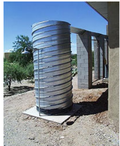
Completed installation of the rainwater harvesting cistern, currently collecting water from flat-roof garage. Photo by Wilson Graham.
