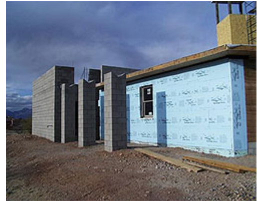
West facade following installation of Dow 2-inch extruded polystyrene insulation over masonry wall.
