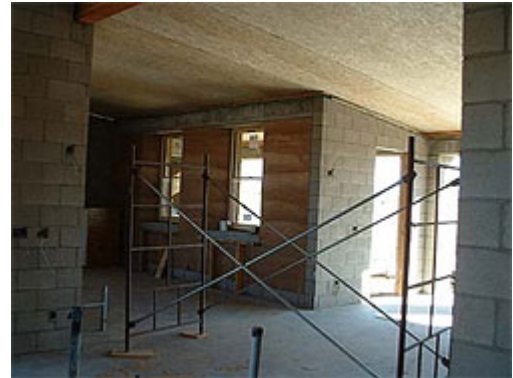
Looking southeast from cooling tower through family room and toward rammed-earth wall and still-unsealed SIPs panels on ceiling. Photo by Wilson Graham.
