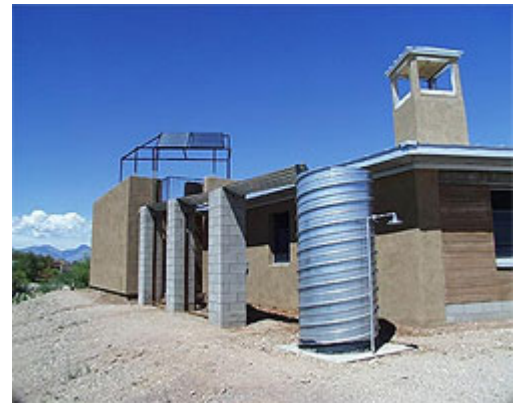
Southwest elevation after installation of the rainwater harvesting aqueduct and cistern and exterior paint. Photo by Wilson Graham.
