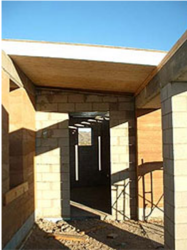
The unfinished southern sun porch, with rammed-earth wall on left and R-38 SIPs panels above guest room. Photo by Wilson Graham.
